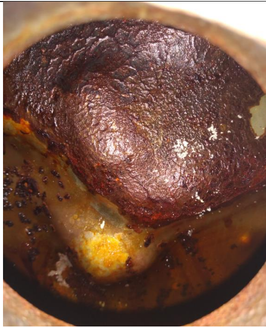
Requires acid wash and re-lining
