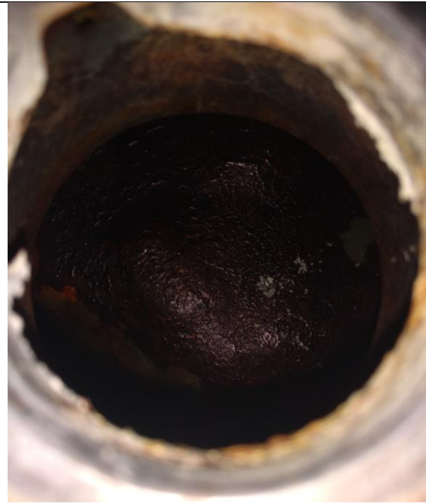
Fuel Tank is rusted
